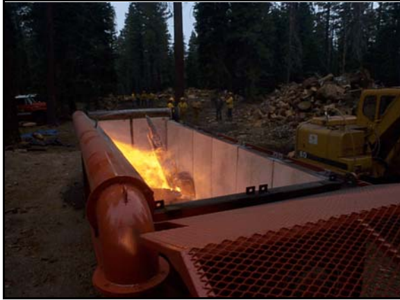
Air Burners S-116, View from Top while in Full Operation with No Visible Smoke, Lake Tahoe, California
