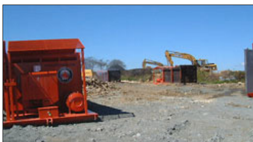
Four S-321& S-116 Units at Disaster Recovery
